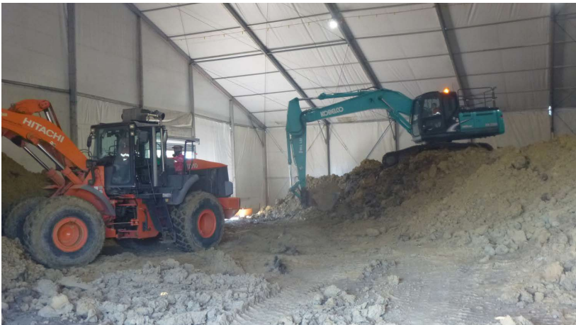
Equipment inside the "tent"
