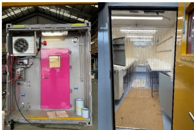
Figures 1 (left) & 2 (right) show the easily recognizable pink door showing the front entrance and through the threshold of the HydroBox during construction.
